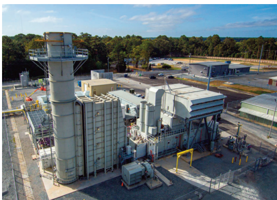
Dominion's Bushy Park CT facility
