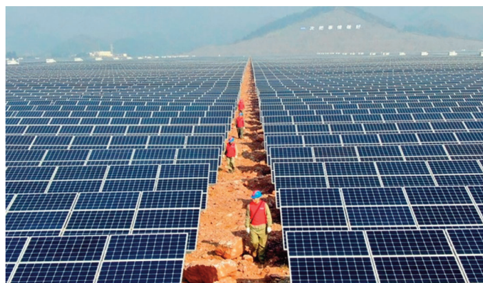
Solar PV installations in Xianning, Hubei province
