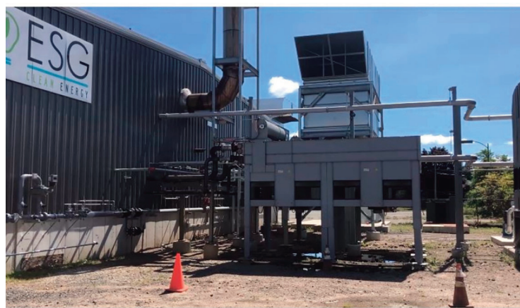
Test plant at Holyoke, powered by CAT gas engines
