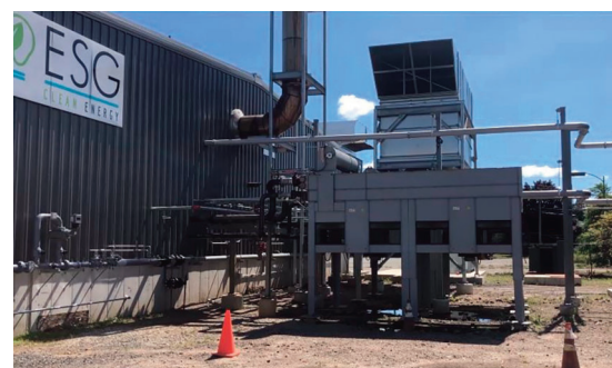
Test plant at Holyoke, powered by Caterpillar gas engines
