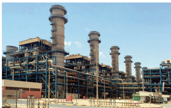
Sabiya power plant near Kuwait City
