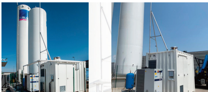
LC3 Trasporti LNG station in Piacenza
