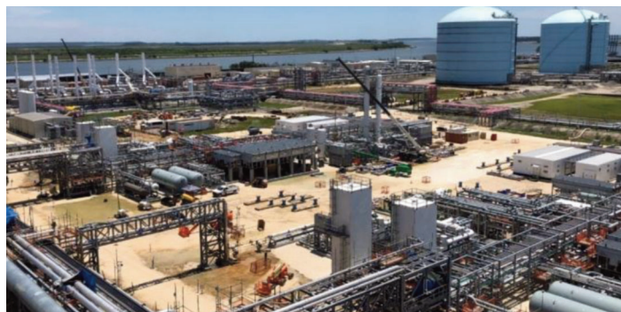
KMI’s Elba Island LNG assets near Savannah in Georgia
