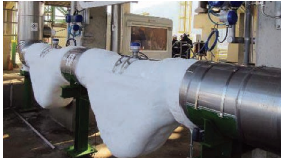
LNG flows should be measured either via Coriolis flow meters or Ultrasonic flow meters
