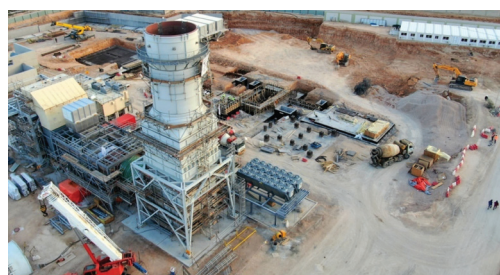
Tobruk open-cycle gas power station in eastern Libya
