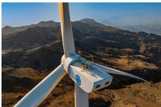
Wind turbine at Al Halah, Fujairah
