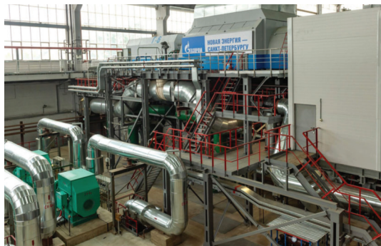
View into Avtovskaya CHP's turbine unit 6
