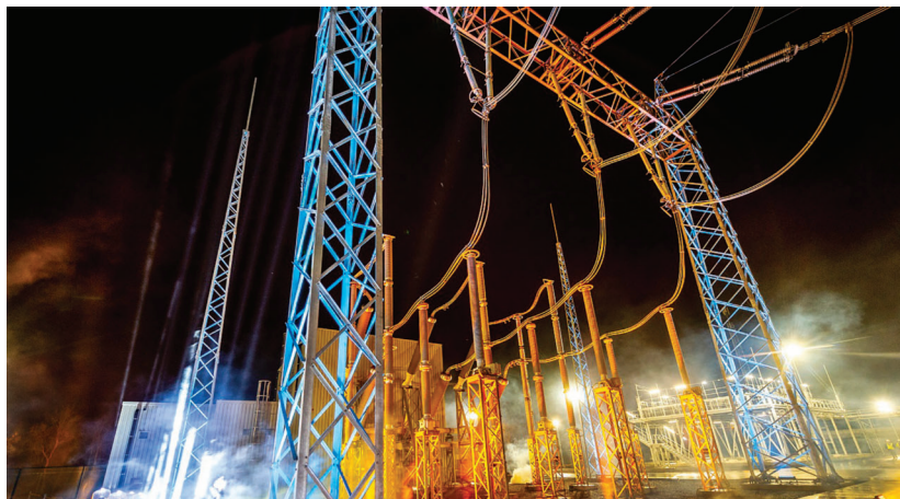
NemoLink, an interconnector between the UK and Belgium
