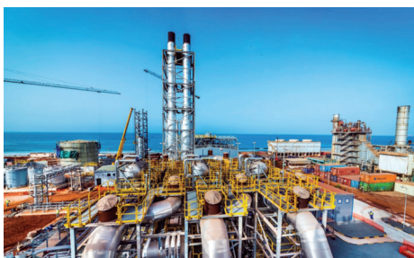
Cap de Biches power plant near Dakar
