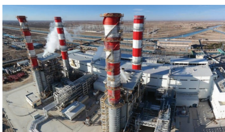
Talimarjan consists of an 800 MW and two 450 MW CCGT units
