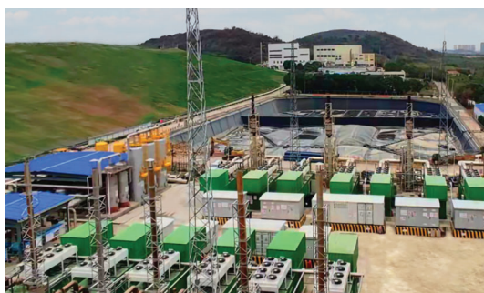
Waste-to-energy plant at a landfill site in Wuhan
