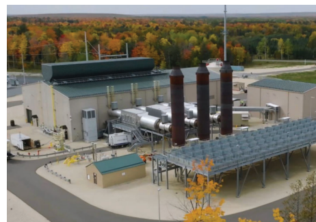
A.J. Mihm power plant during testing
