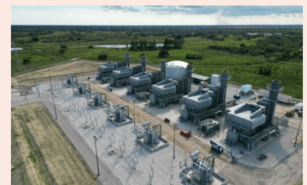
Mark One Generating Station
