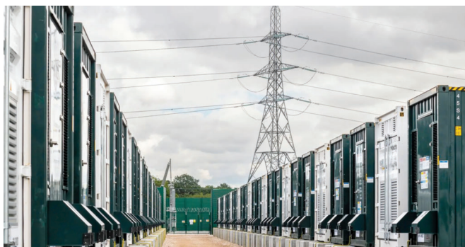
Zenobē's Capenhurst BESS in Chester
