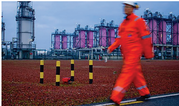
Receiving terminal for Norwegian gas at Emden, Germany.
