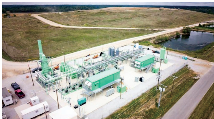
RNG plant at Medora is next to a landfill owned by Rumpke
