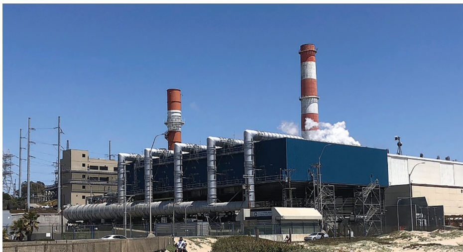
View of Scattergood Generating Station near LA
