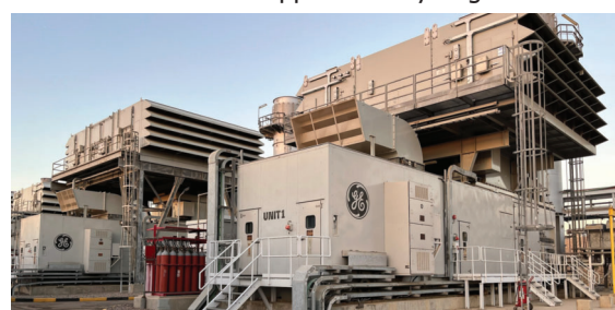
EEHC's Sharm El Sheikh power plant
