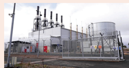
Brigg gas peaking plant in Lincolnshire
