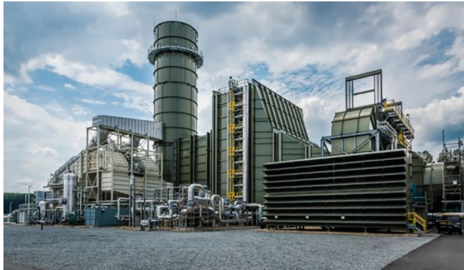
Duke Energy's Lincoln SCGT near Charlotte, North Carolina
