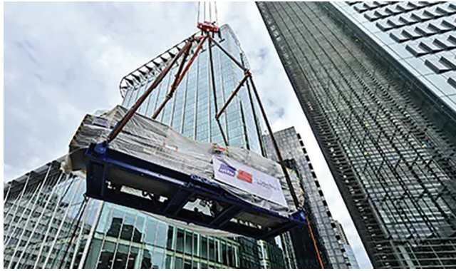
mtu genset being installed at a high-rise in London
