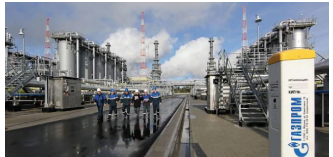
Portovaya compressor station on the Russian entry point of Nord Stream 1
