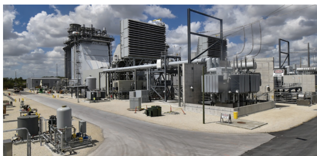
Dania Beach Clean Energy Center
