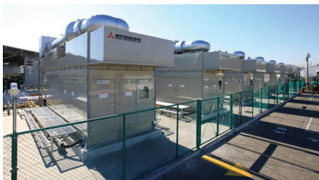
Gas engine generator sets in MHIET's Sagamihara Plant
