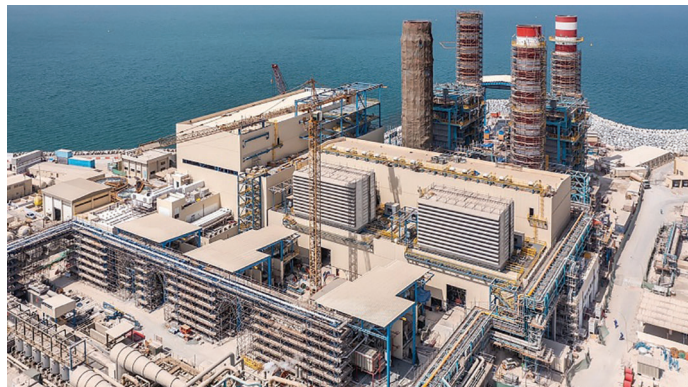
SEWA's Al Layyeh power plant expansion
