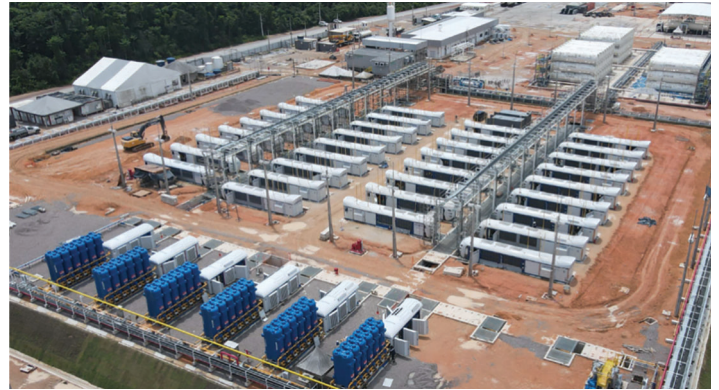
Galileo Technologies installed at one of H&P drilling sites in the US
