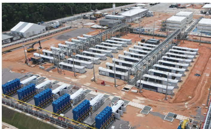
Galileo Technologies Cryoboxes set up at Azulao field owned by Brazilian utility Eneva
