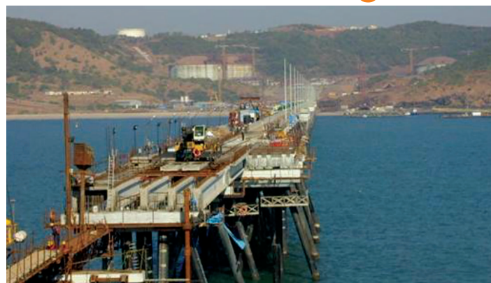
Dabhol terminal in Maharashtra state south of Mumbai
