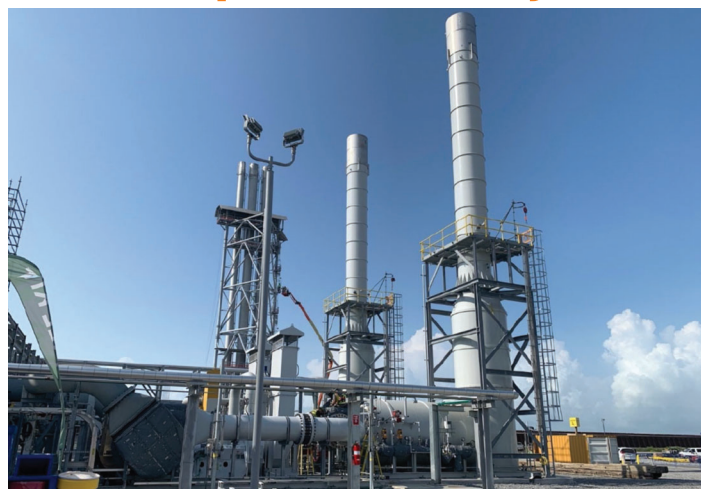
Thermal oxidizers are among growing equipment array
