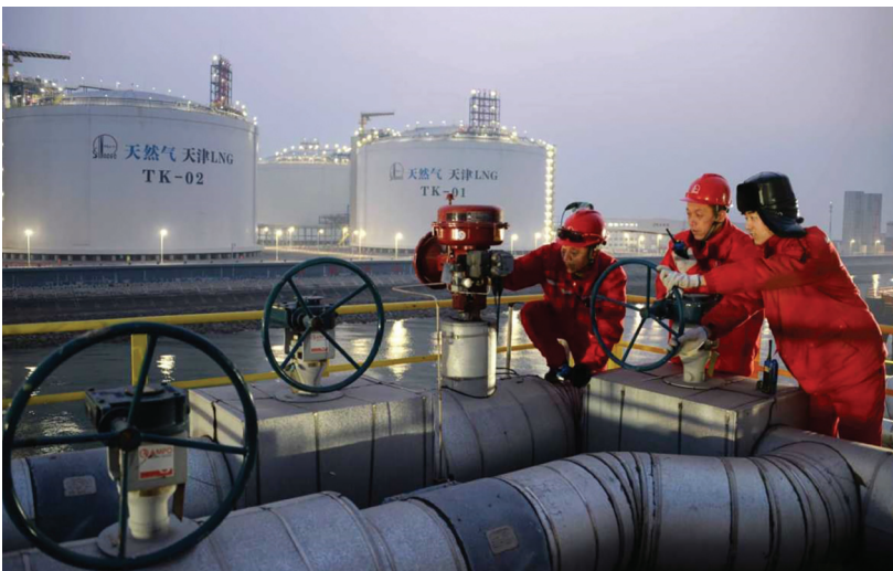
Sinopec technicians check LNG facilities in Tianjin.
