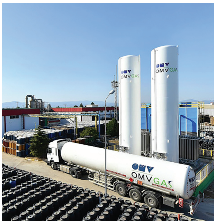
OMV Gas facility
