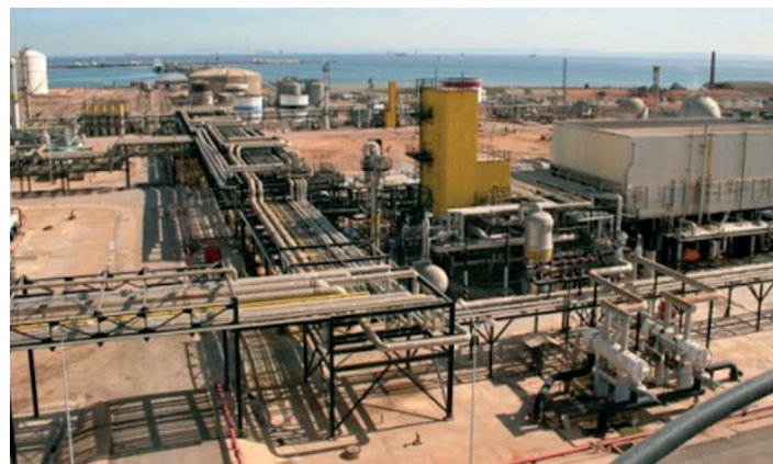
Sonatrach's LNG facility at Arzew on Mediterranean coast
