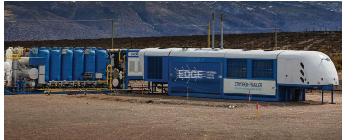
Truck-delivered LNG equipment includes Cryobox liquefaction for Edge-Exco Resources project
