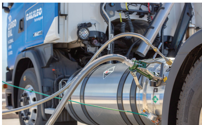
LNG dispenser connected to the trucks cryogenic tank
