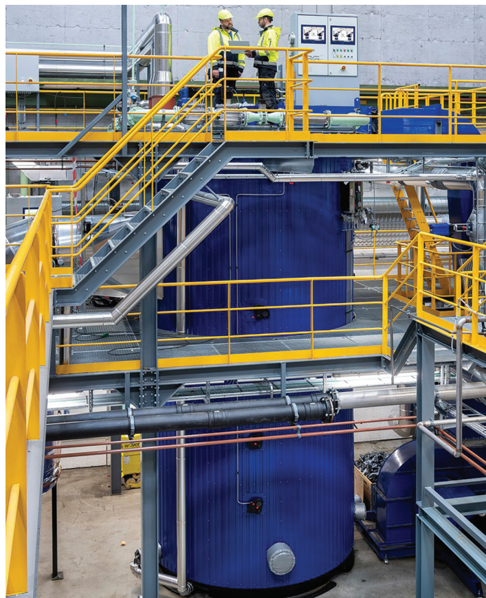
An Aalborg boiler seen on test
