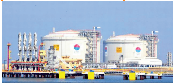
Petronet's import terminal at Dahej, north of Mumbai
