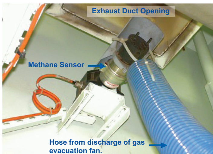
The unauthorised arrangement
