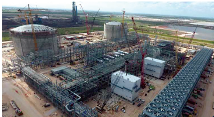
Texas export plant is located on shore of Corpus Christi Bay
