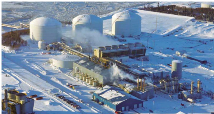
Existing Kenai LNG plant owned by ConocoPhillips
