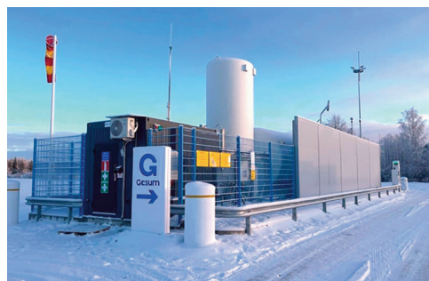
Ylivieska bioLNG filling station
