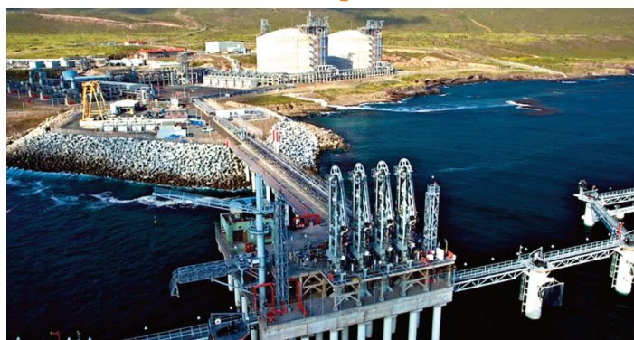
Sempra's ECA LNG receiving terminal
