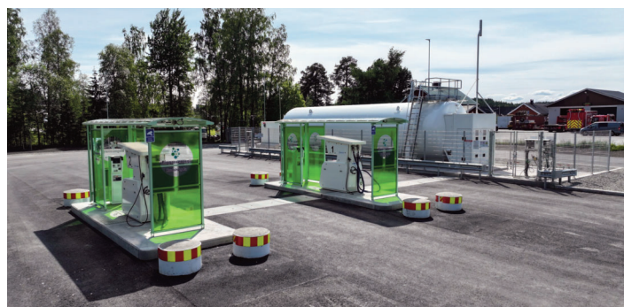
Biogas Energi refuelling station
