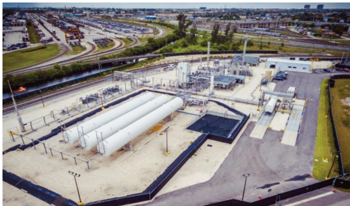
Liquefaction plant processes 100,000 gallons of LNG a day
