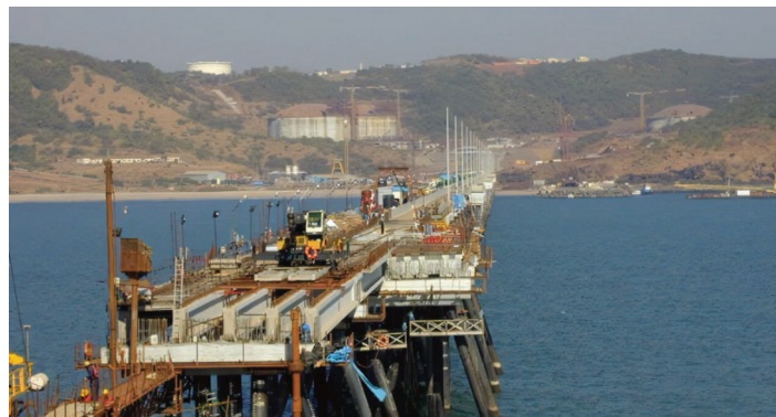
Unloading jetty for GAIL's Dabhol import terminal
