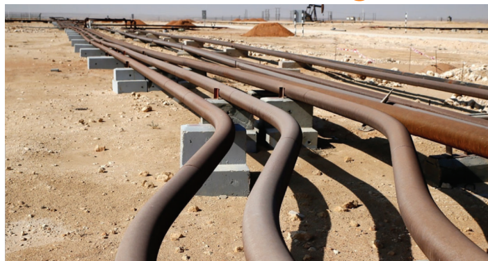
Oman Gas Networks has around 4,000 kilometres of pipelines with its concession lasting for 70 years
